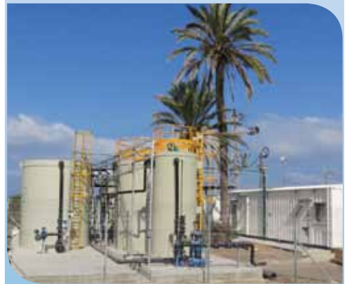
Well water treatment–Israel (1,300 m 3 /d)
